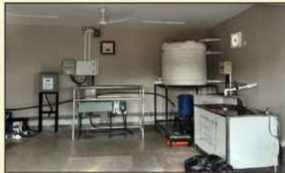
Internal Set-up of the Biogas plant
