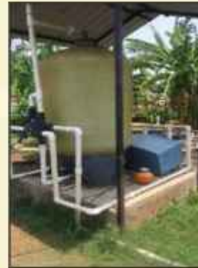
Filtration plant for rainwater
