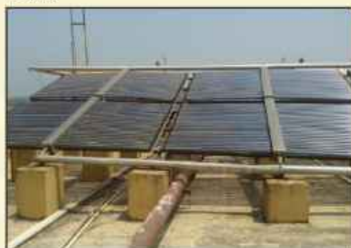
Solar water heating system
